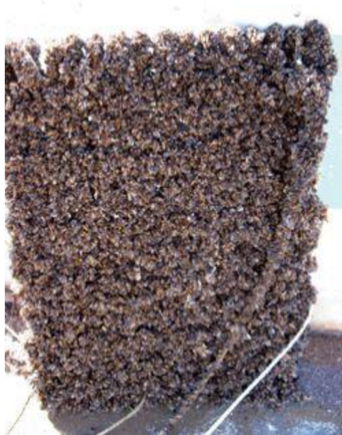
Quagga and zebra mussels completely clog a steel grate in just seven months.
